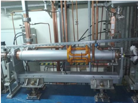
Fig. 5. NSC KIPT corrector installed at the accelerator section
