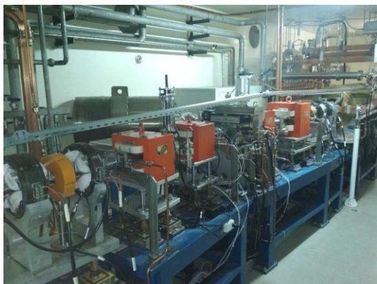
Fig. 11. Electromagnetic chicane with installed dipole magnets CB1-CB4, electron beam collimator and electron beam energy measurement channel
