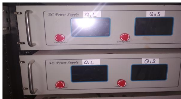
Fig. 33. Power supply source without water cooling
