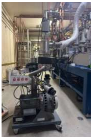
Fig. 18. Preliminary pumping mobile unit
