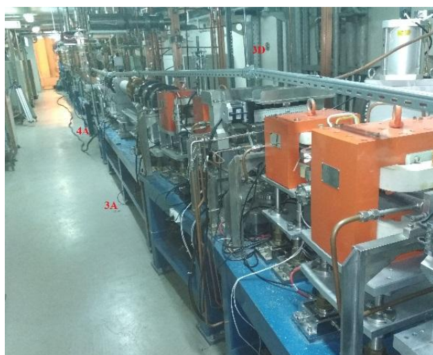
Fig. 14. The view of the accelerator equipment allocation in the facility 100 MeV/100 kW accelerator tunnel and target-reflectors of the accelerator tunnel geodesic network
