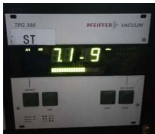
Fig. 15. Vacuum monitor panel in the klystron gallery cabinet
