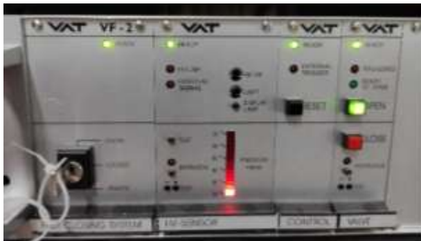
Fig. 11. Fast valve control unit
