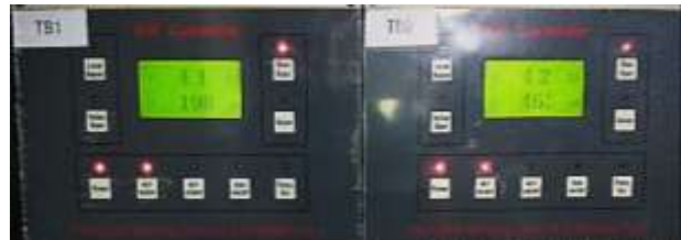
Fig. 20. TB-1 and TB-2 in operation
